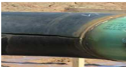
Fig. 2. Crack propagation in pipeline
